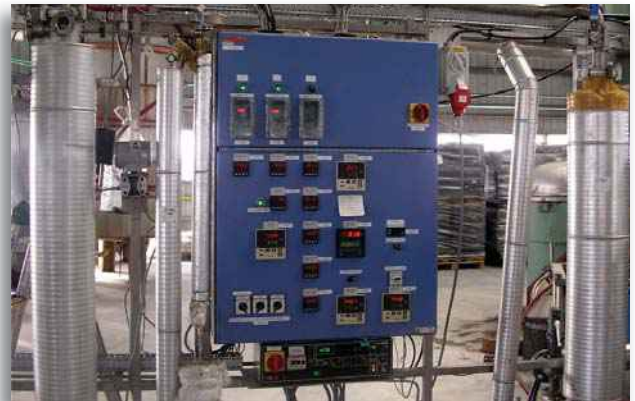
Partial view of the olive pomace oil production plant yielding oil with a high concentration of triterpenic acids.
