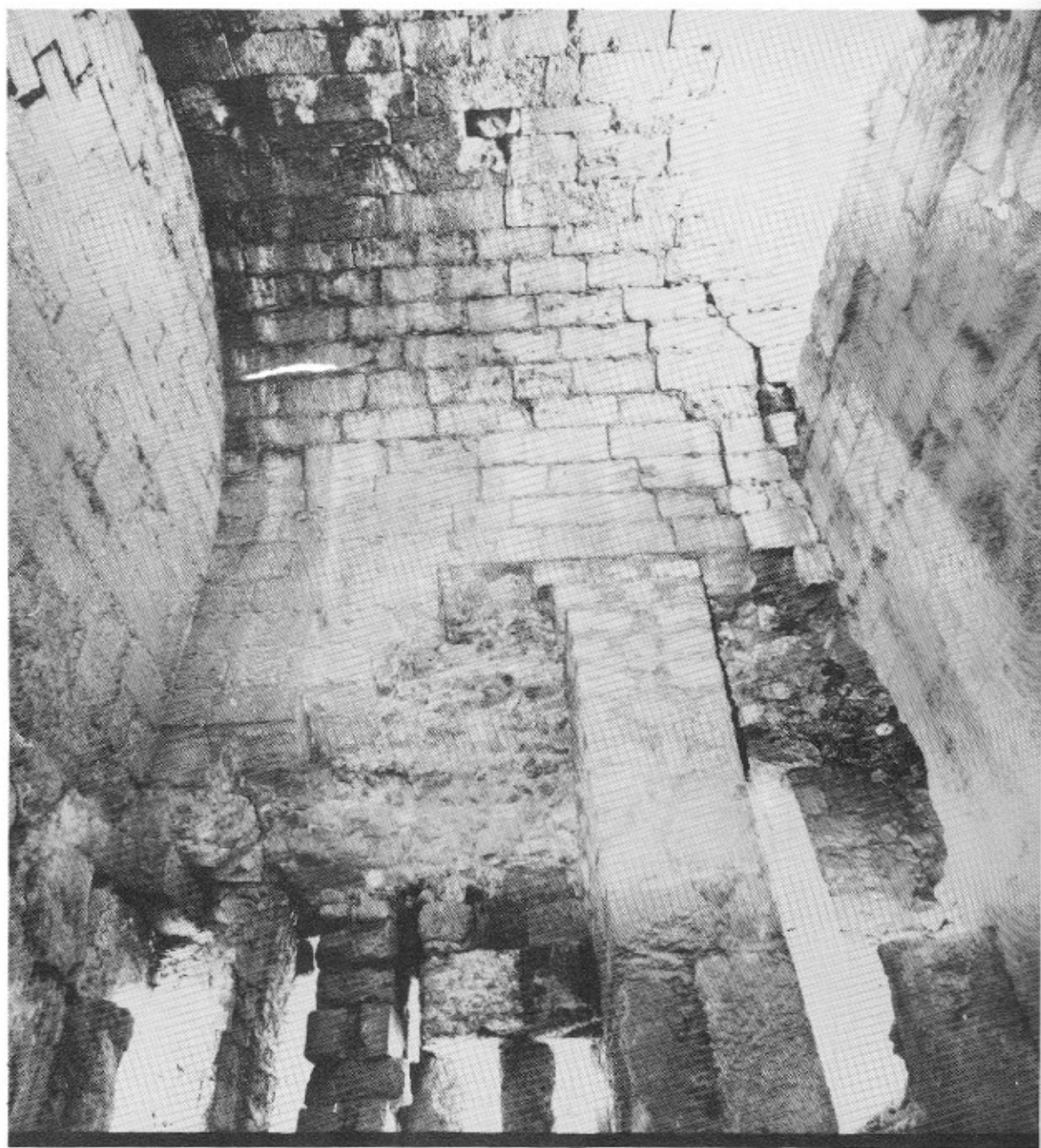
Fig 3: The west wall of the northeast room before the restoration.
