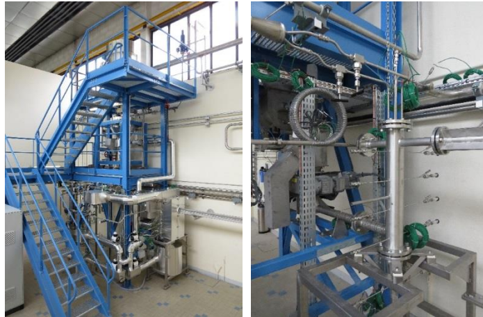
FIGURE 7. Photo of the insulated facility (left) and of the BFB reactor (right)
