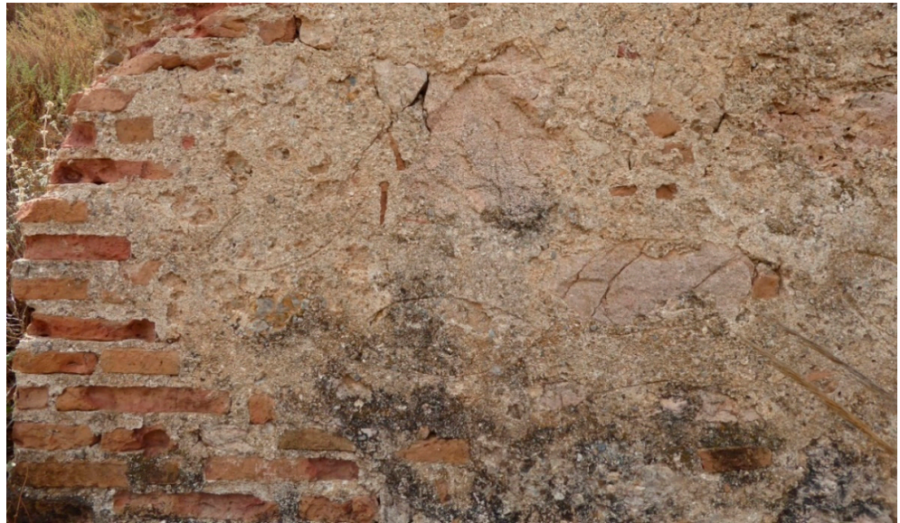
Figure 10. North side of the tower gate, Mondújar Castle. In this picture, the fish-like incised lines, made on the lime mortar plastering, can be appreciated (Antonio Orihuela, 2020).
