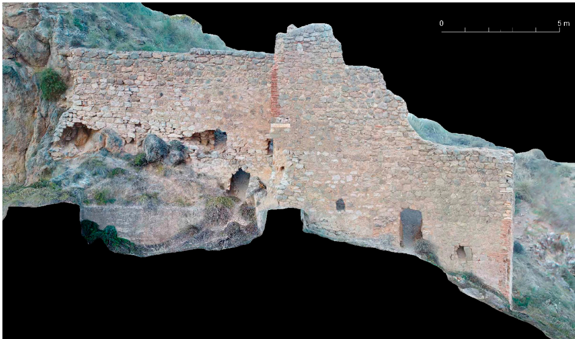
Figure 8. Orthophoto of the north elevation of the Castilian fortress, Mondújar Castle (Antonio Orihuela; Víctor Martín-Madrid, 2020).
