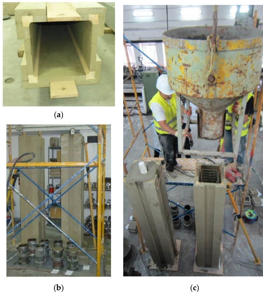
Figure 2. Cast process of the specimens: (a) Detail of a wooden formwork with rounded corners; (b) General view of two wooden formwork and cylindrical normalized specimens; (c) Cast process.
