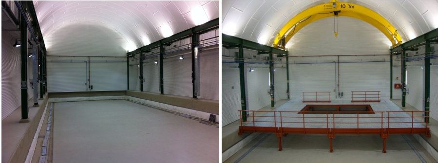
Figure 9.2.8: View of Hall A of the Laboratorio Subterráneo de Canfranc prior to any equipment installation (left). Hall A with the working platform already installed (right). Installation of the seismic infrastructure will be ready in 2014.
